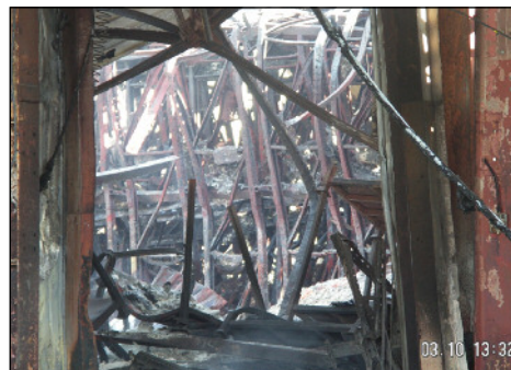
The fire in this case was hot enough to melt the steel girders, creating this dramatic looking scene.
